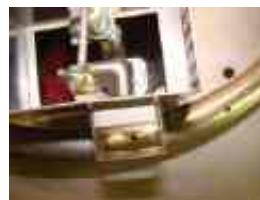
Top View- note next to burner
